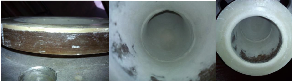
This fitting pictured above was just off the pump discharge.
